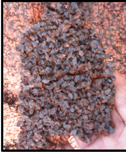
TRACK SURFACE DELAMINATING
