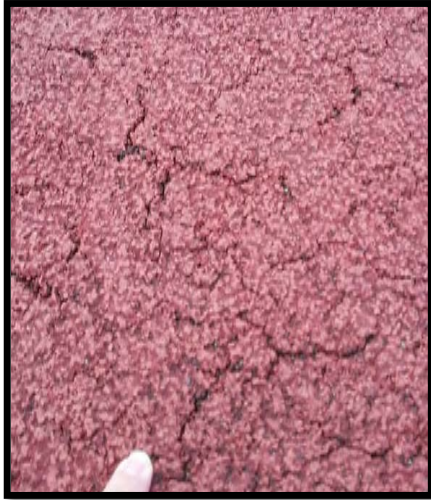
TRACK SURFACE CRACKING
